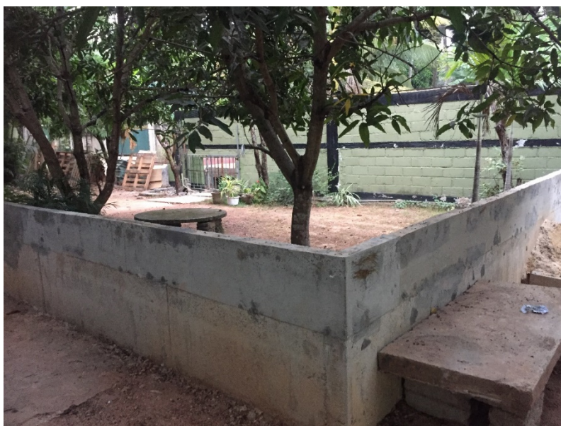
Picture 5 New wall built in Gampaha SME unit to block flood waters
