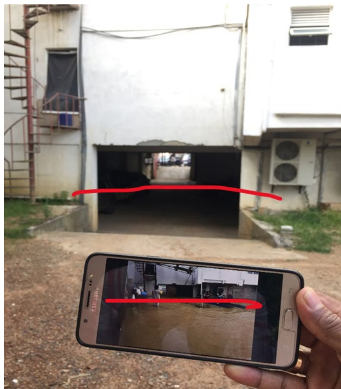
Picture 4 Flood levels during a recent event
